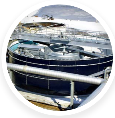
Municipal Wastewater Clarifier / Sludge / Storage / Mixing
